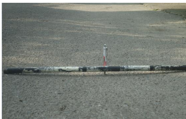
Fig 5: Rutting on an asphalt pavement
