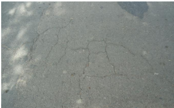
Fig 4: Fatigue cracking on an asphalt pavement
